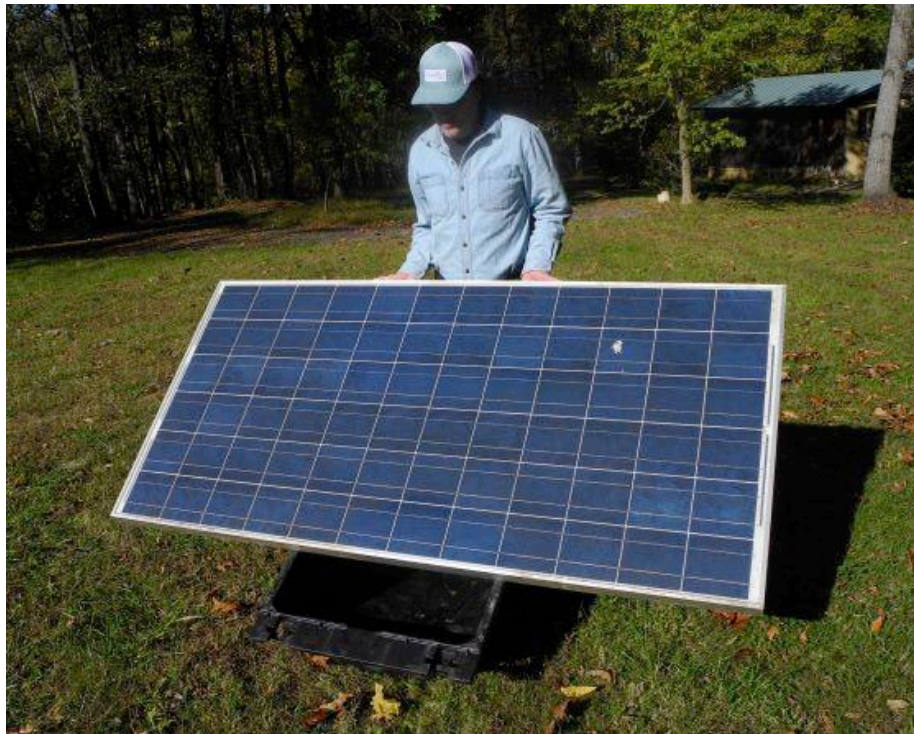
Figure 12. Worker resting panel on the PowerRack side rails ready to slide into place.
