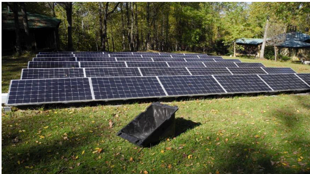
Figure 2. PowerField PV Solar Array
