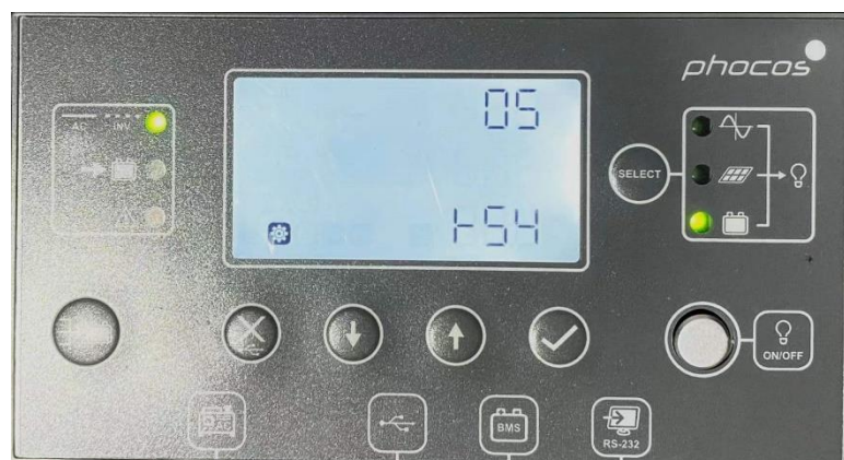
Figure 2.1.2.5 Phocos inverter battery type selection
