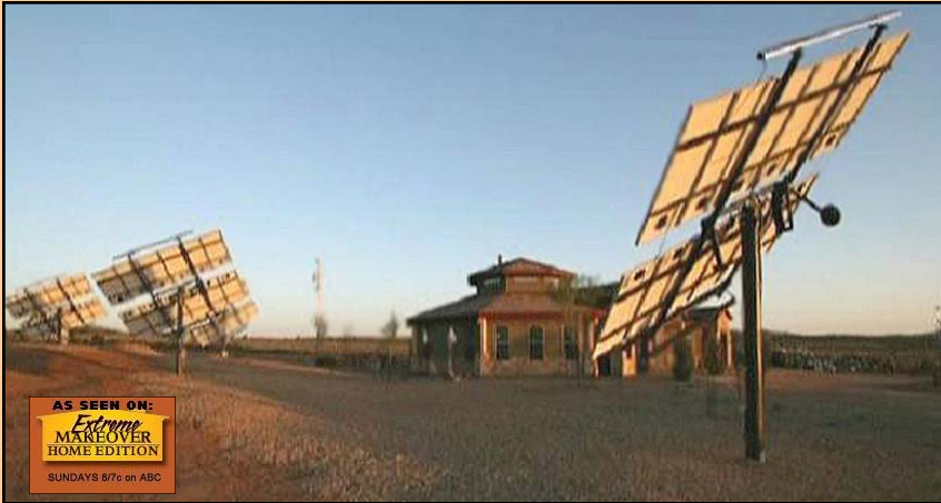
ABC EXTREME MAKEOVER "YAZZIE FAMILY" HOME FEATURING ZOMEWORKS UNIVERSAL TRACK RACK™ MODEL UTRF-168 "THE EARLY BIRD'S VIEW" INSTALLED BY MARK SNYDER ELECTRIC
